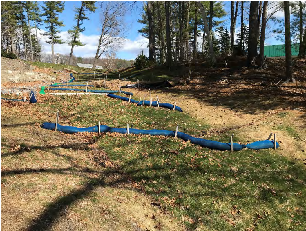
Fig 10: Slope below the manhole at Gundalow Landing/east side of the bay. Viewing east. (04-06-21)
