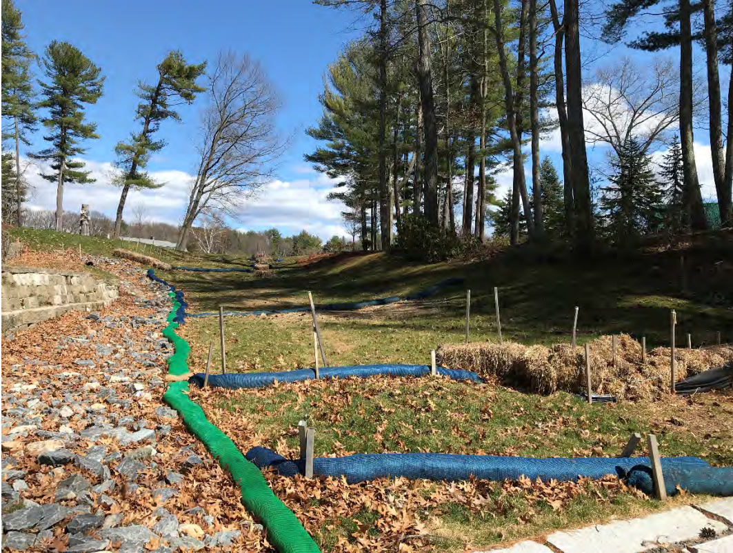
Fig 9: Slope above the manhole at Gundalow Landing/east side of the bay. Viewing east. (04-06-21)
